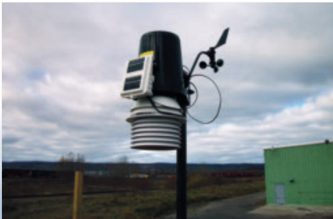
WEATHER DATA TRANSMITTER — These photos (above and right) show the weather data transmitter installed in the AGGRAND growth plots.
